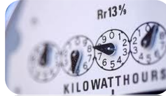
Energy Metering (Gas, Water, Electric)
